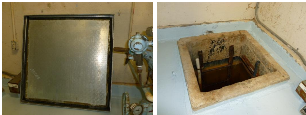
Contact chamber with adequate gasket on reservoir hatch and contact chamber opening
