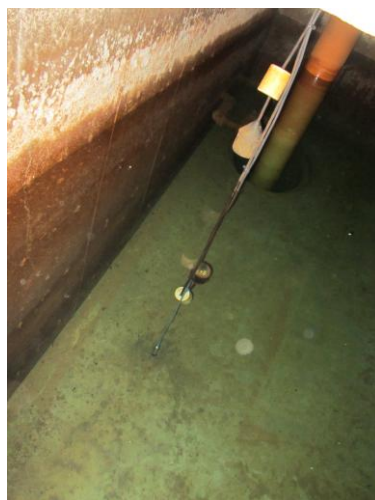
Midway reservoir floats and pressure transducer
