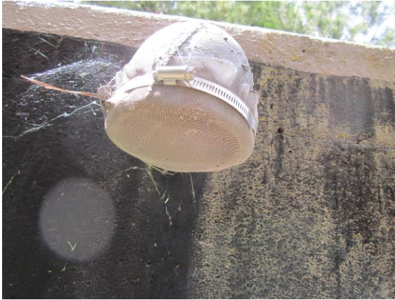
Upper reservoir vent/overflow
