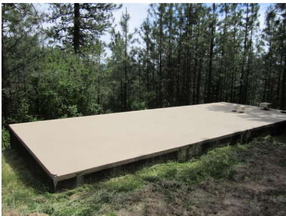
30,000 gallon upper reservoir
