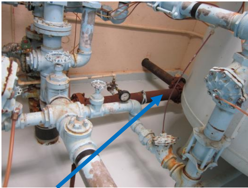
Raw water feed line to plant
