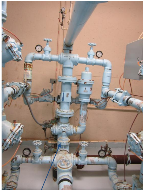
Raw water connection with pre-filtration feed line
