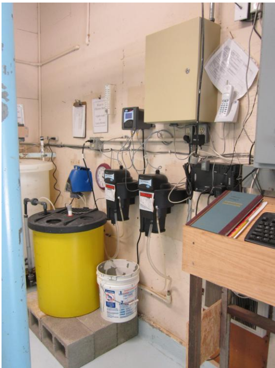
NaClO day tank and metering pump 1720E individual effluent turbidimeters
