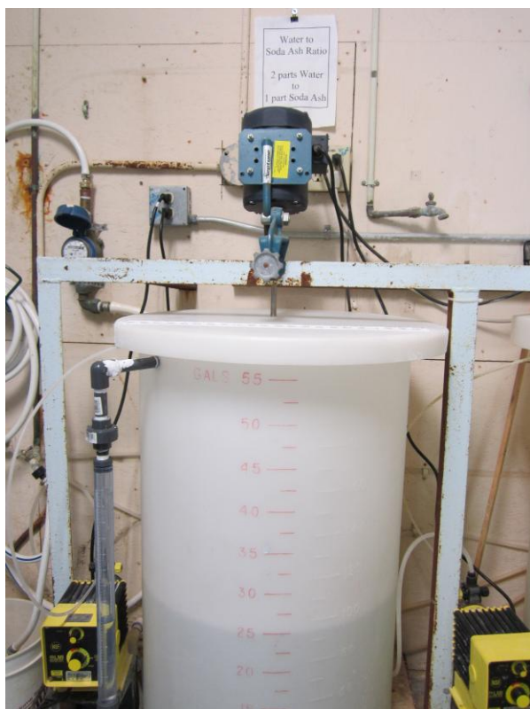
Soda ash injection system
